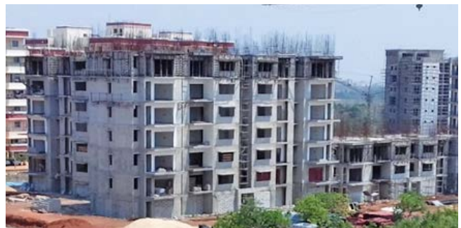
Type-C1 & C2 Quarters: C1- 5 th floor roof slab Completed and C2 - 2 nd floor roof slab completedc
