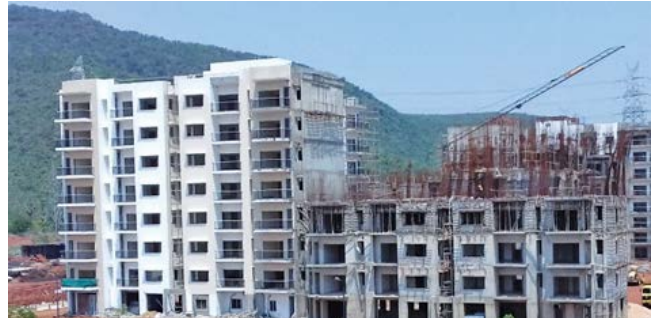
Type-B1 & B 2 Quarters: B1 finishing work is in Progress and B2- 2 nd floor roof slab completed.
