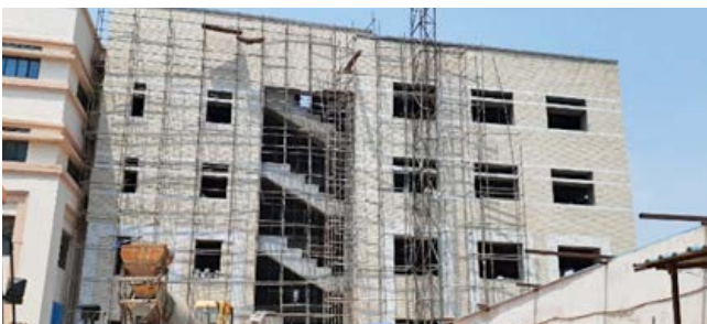
SES Extension (B- Wing): The structural work completed & finishing work is in progress
