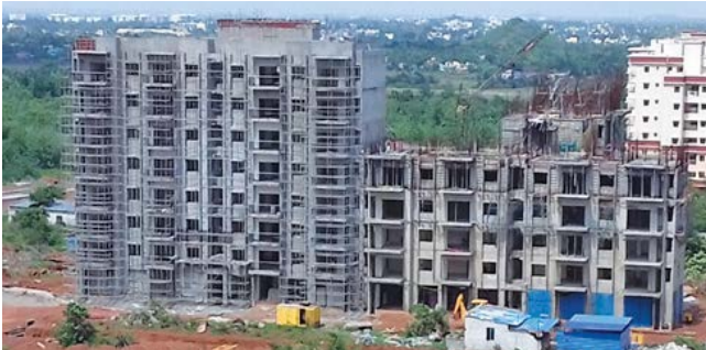
Type-A1 & A 2 Quarters: A1 finishing work is in progress and A2- 3 rd floor roof slab completed.
