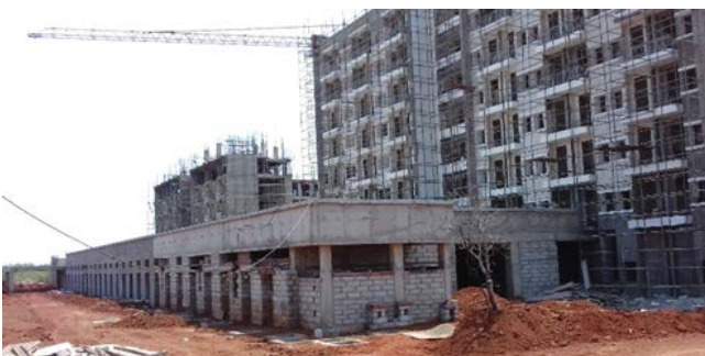
Boys' Hostel-3: Front side dining and multipurpose hall Finishing work is in progress.
