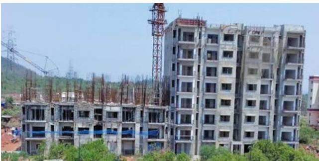
Type-B3 & B 4 Quarters: B3 - 2 nd floor roof slab completed and B4- finishing work is in progress
