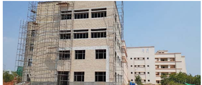
SES Extension (A- Wing): The structural work completed & finishing work is in progress
